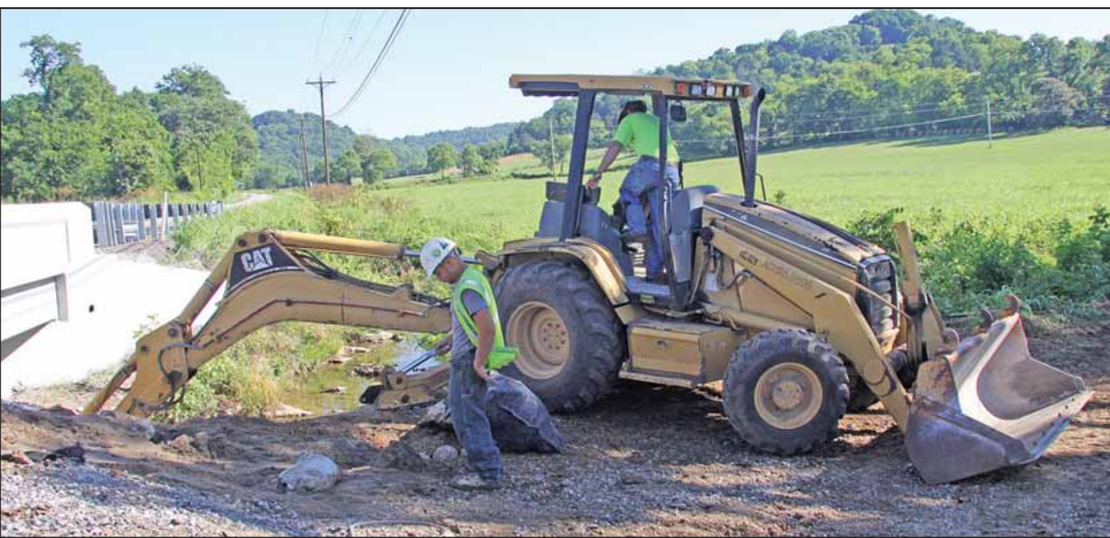
Putting on the finishing touches on the new Rush Creek Bridge between Woodbury and Auburtnow, the new bridge was completed in 21 days from start to finish.
